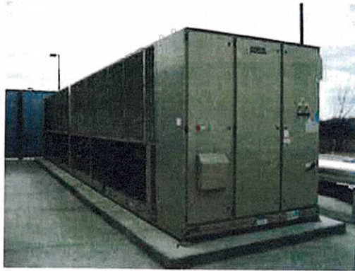
McQuay Chiller AWS400 Model
