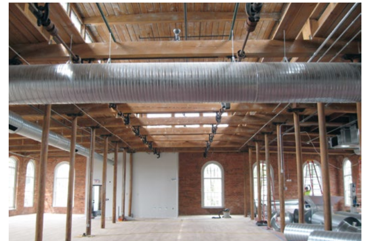
[39] Leaving the ceiling structure exposed and installing exposed ductwork where it does not impact the windows, are appropriate treatments when rehabilitating an industrial building for another use.
