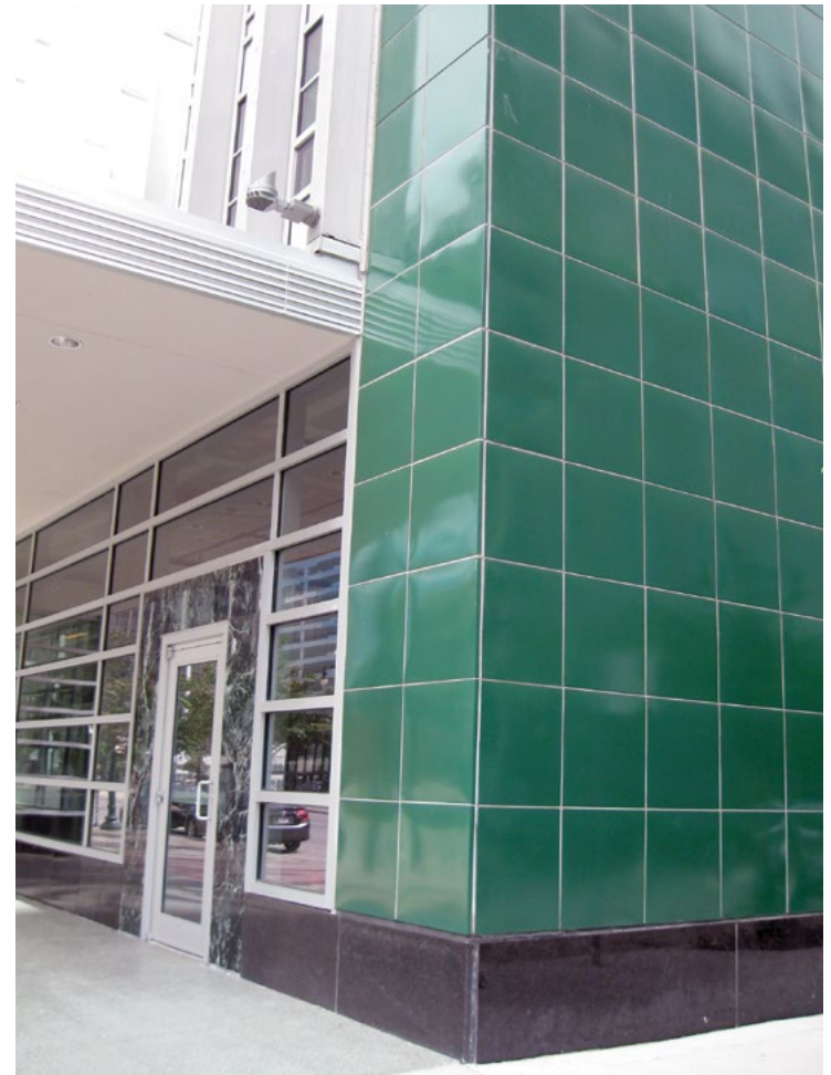
[15] New enameled-metal panels were replicated to replace the original panels, which were too deteriorated to repair, when the storefront of this early 1950s building was recreated.
