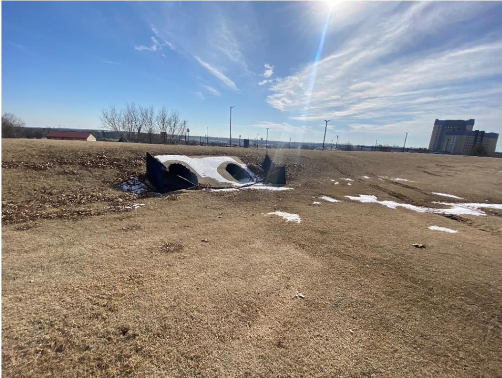
Figure 6: Underground drainage feature noted near boring P-02
