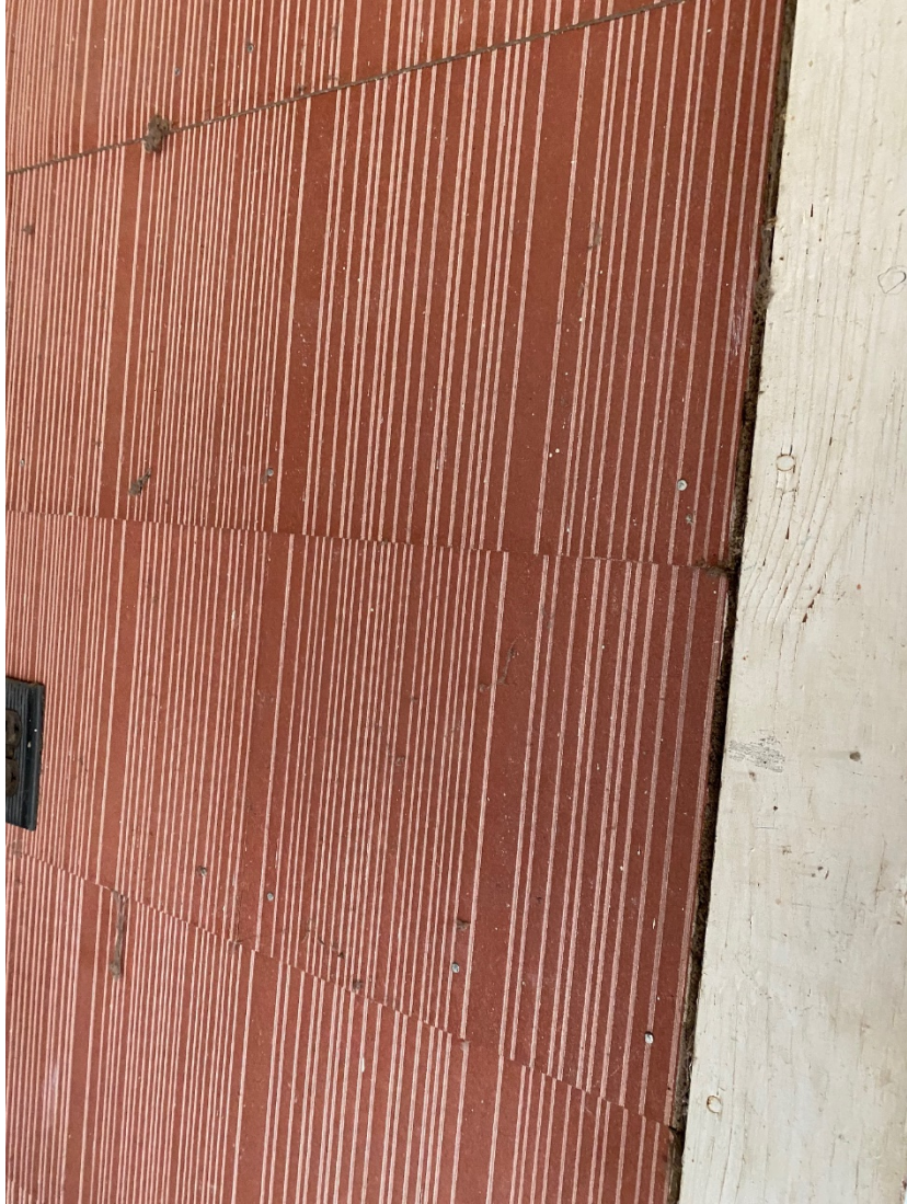
Photograph 3: Exterior Siding 20% Chrysotile Asbestos
