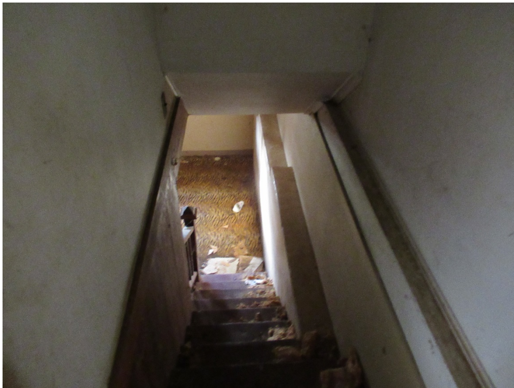
Photograph 2: 9x9 Floor Tiles below carpet on lower level, 4% Chrysotile Asbestos
